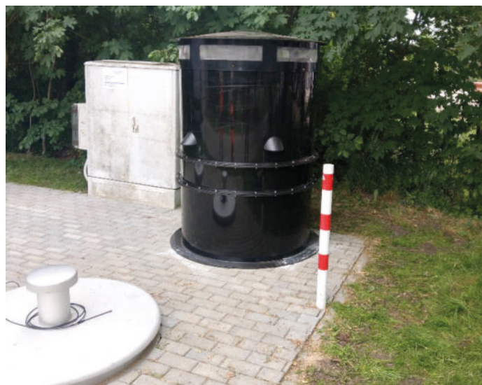
Filter for removing odour from exhaust gas in a sewage tunnel
